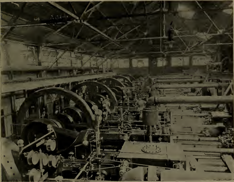
Interior of Manhattan Air Compressor Plant, P. R. R. East River Tunnels.
